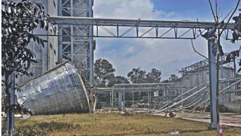
The damaged gas tank and pipes of DAP Fertiliser Company Limited in Anwara upazila of Chittagong. An explosion at the factory on Monday night caused the damage. Photo: Anurup Kanti Das
